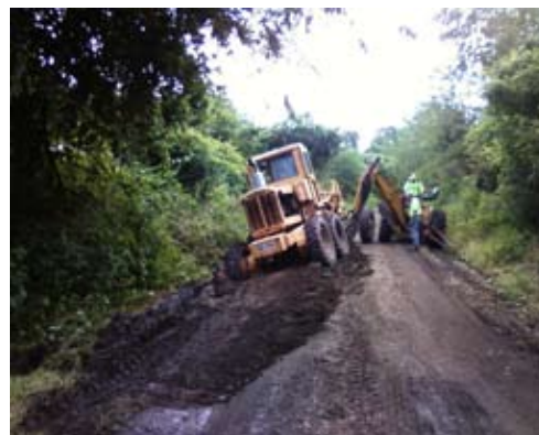
Bill Capp checks over Frank Ludwin's grading and digging. (Photo- John Kozak)
