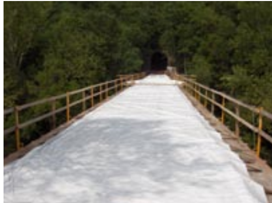
The deck for the Chartiers Creek Bridge was poured on Friday, July 11 lying in place as it cures. Photo by Troy Bogdan
